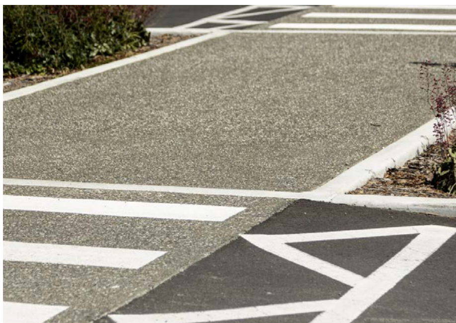
Exposed aggregate pedestrian crossing NOTE: Ensure exposed aggregate used at zebra crossing provides adequate contrast to line marking.
