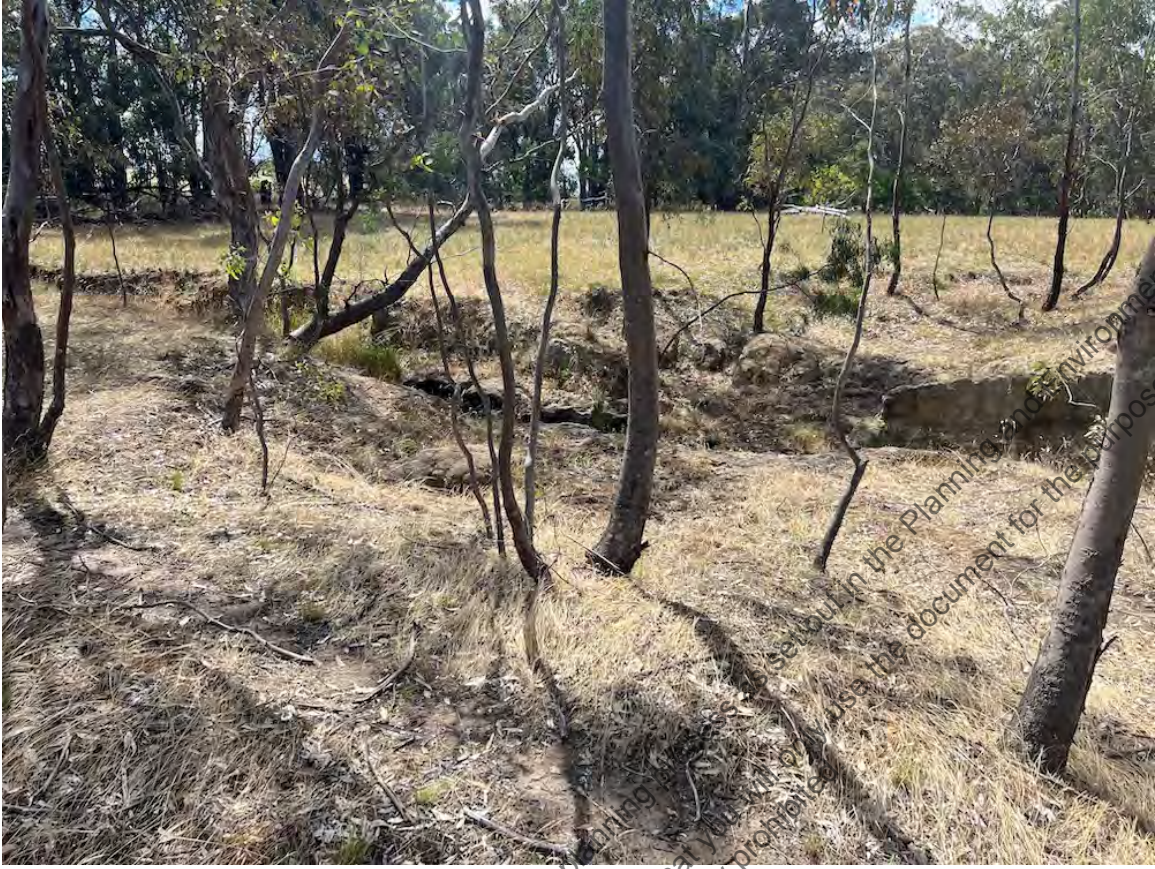
Figure 55 – Stable erosion with regenerating overstory on Lot 2
