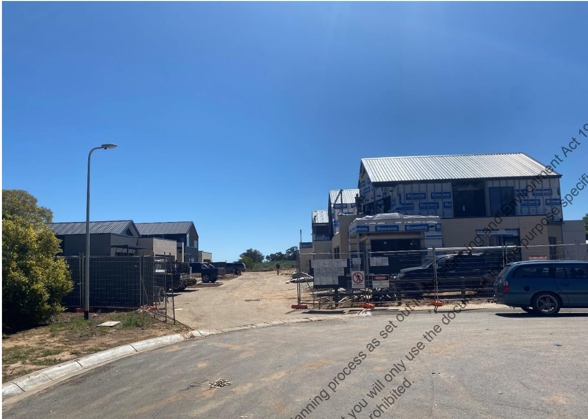
Figure 19 - Double-storey development under construction at the end of the River Street courtbow
