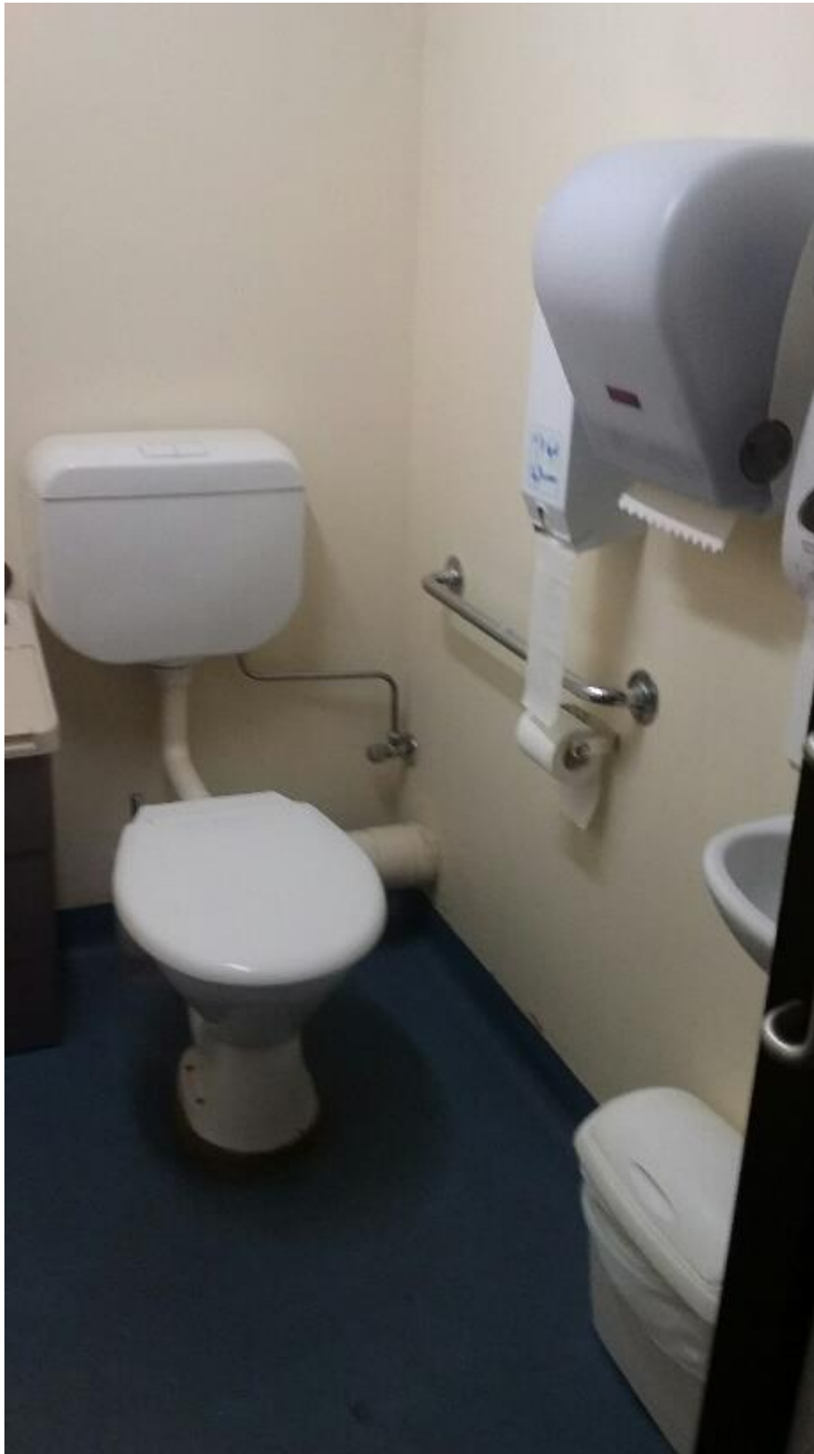
Inside the accessible toilet
